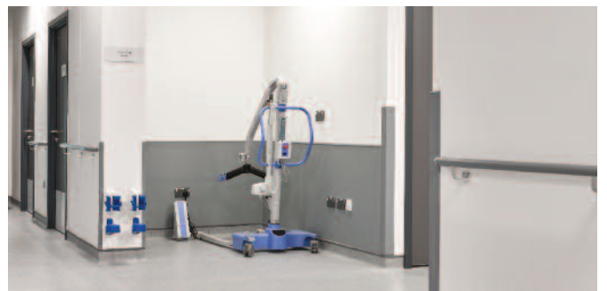
Rubber wall and corner guards have been fitted to protect back-of-house areas in the hospital against damage from wheeled equipment.
